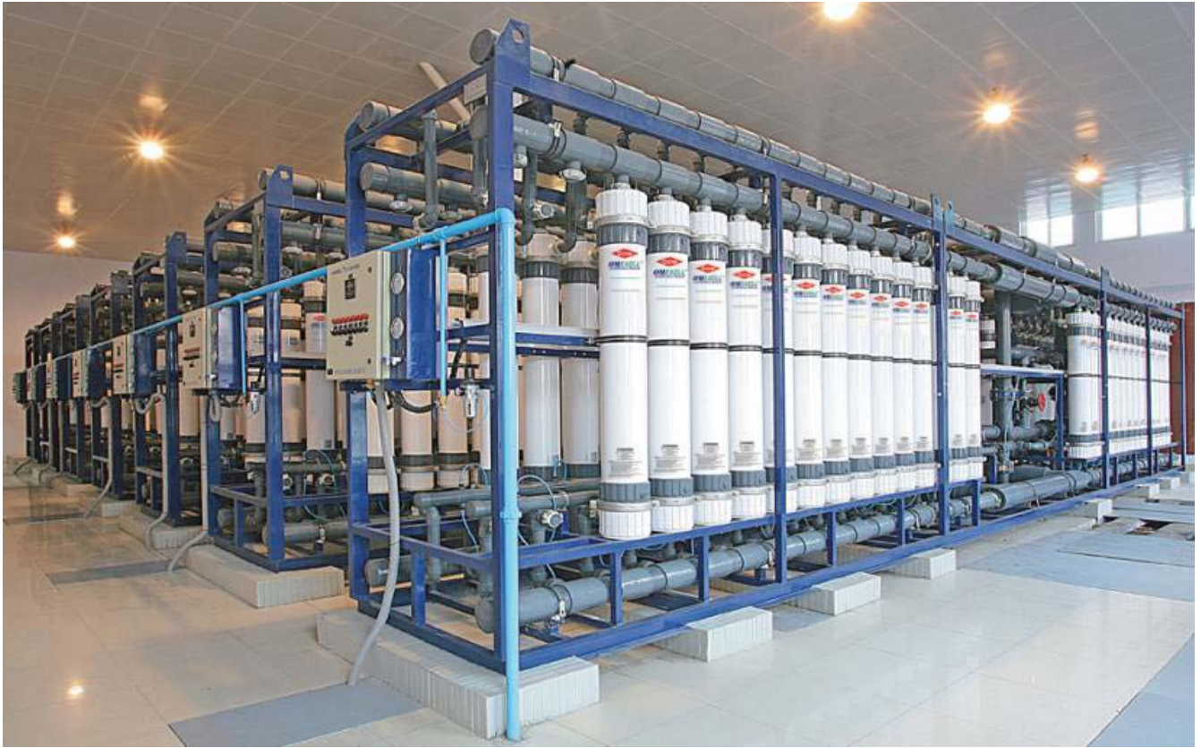
Figure 9: DOW UF Installation using 2860 Modules
